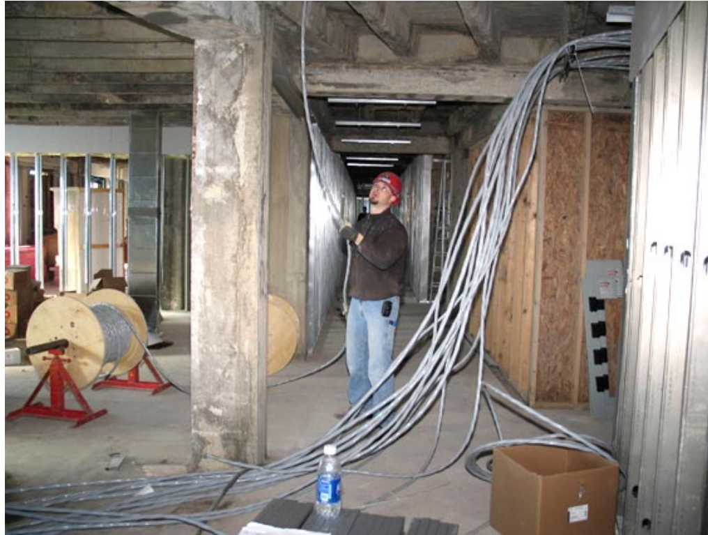
FEEDING NO. 2 WIRE up to the seventh floor of the Durant Hotel in Flint is Aaron Allen of IBEW Local 948, working for Goyette Mechanical.
