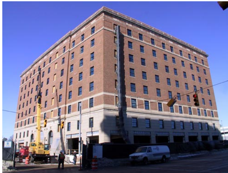
COMPLETED IN 1920 – the start of an automotive boom era for the City of Flint – the Durant Hotel will reopen this year as an apartment building that would appeal to students at the nearby U-M Flint campus. The first floor lobby and ballroom will be restored to their original appearance, while upper floors have been
